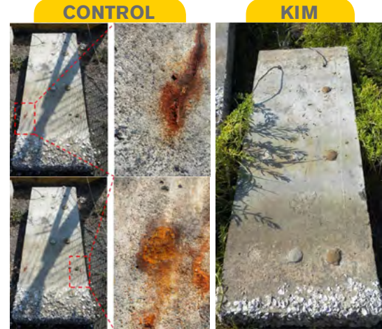
After 10 years marine exposure; Control concrete / KIM treated concrete.
