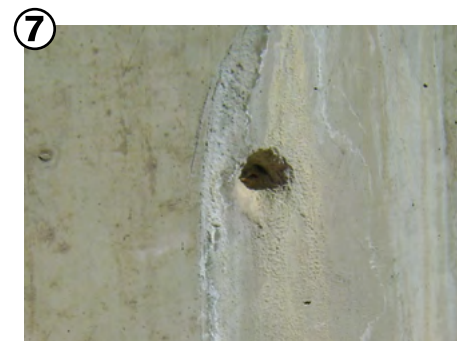
Repair leaking pipe penetrations and tie holes with Krystol Leak Repair System.
