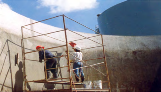
Annacis Island Wastewater Treatment Plant, Vancouver, British Columbia, Canada
