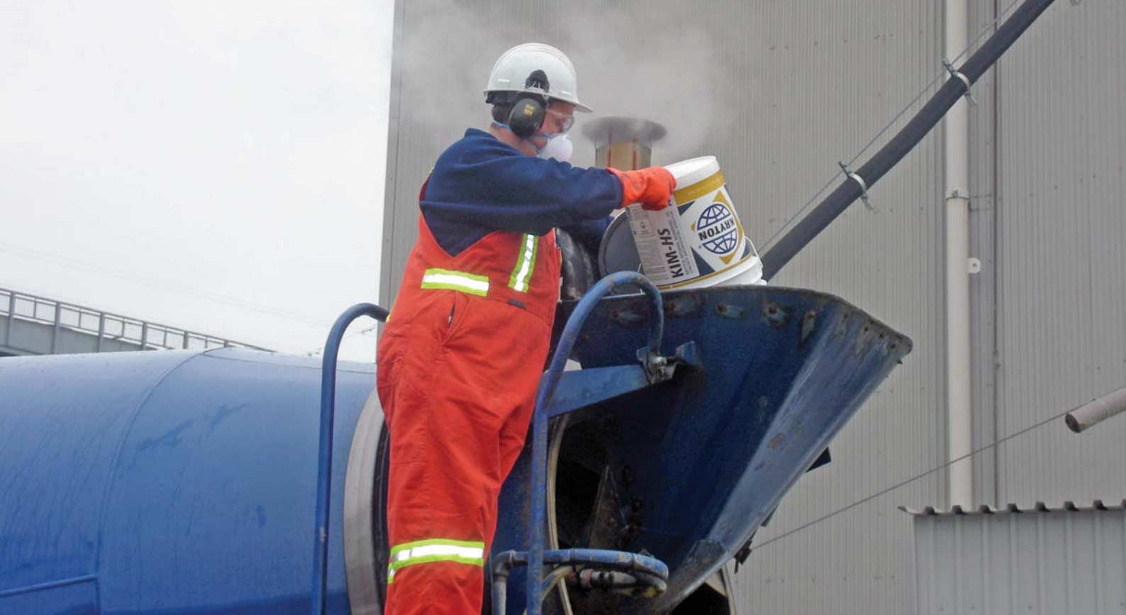
KIM admixture is added to ready-mixed concrete truck at time of batching.
