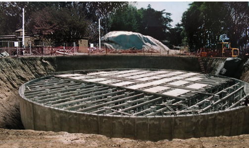
TreePeople Center Rainwater Cistern, Los Angeles, USA
